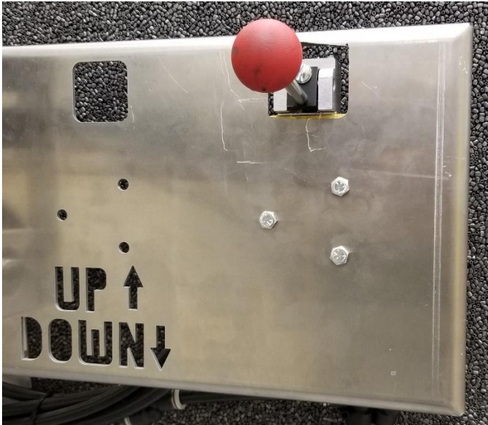
Pneumatic controls for Class 1 Div. 1 environment. And cut out decals.
