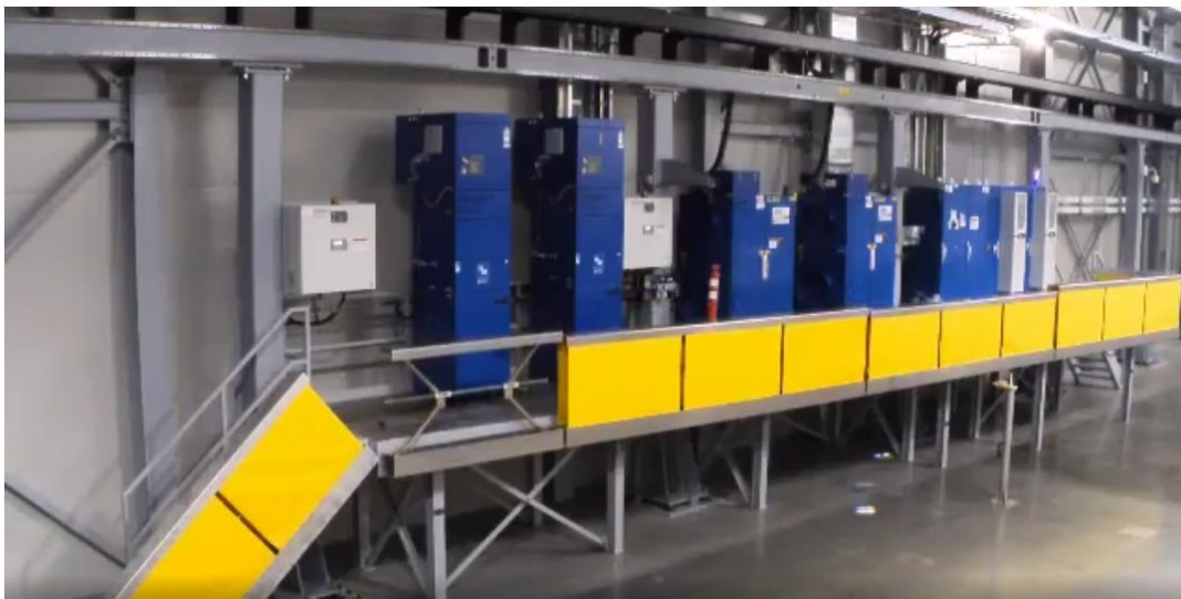
Fully Integrated , with PLC and HMI controls.
