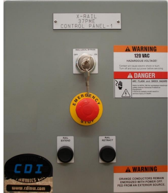
Electrical controls for factory environment with keyed supervisor override switch.
